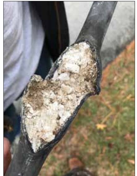
Since Hurricane Florence, Tideland crews are more frequently encountering corroded underground powerlines like the one above.
